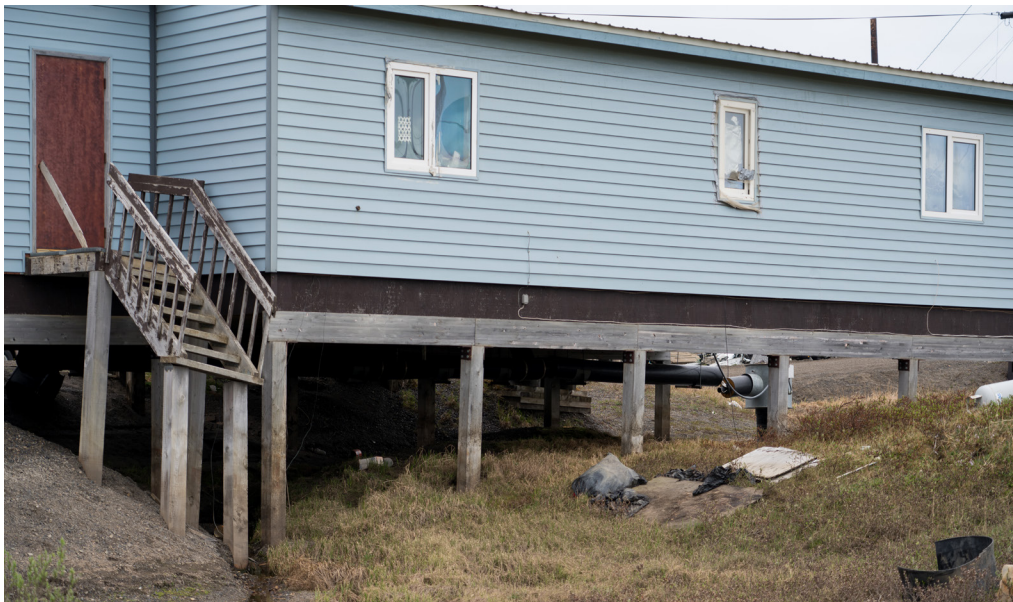
Figure 23. Example of Stair Conditions and Damage. (Point Lay Resident Bill Tracey, 2022)
