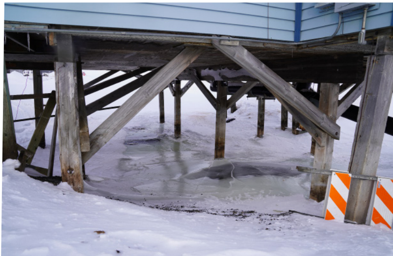
Figure 4. Frozen Pooled Surface Water Below Home. (NREL, 2022)
